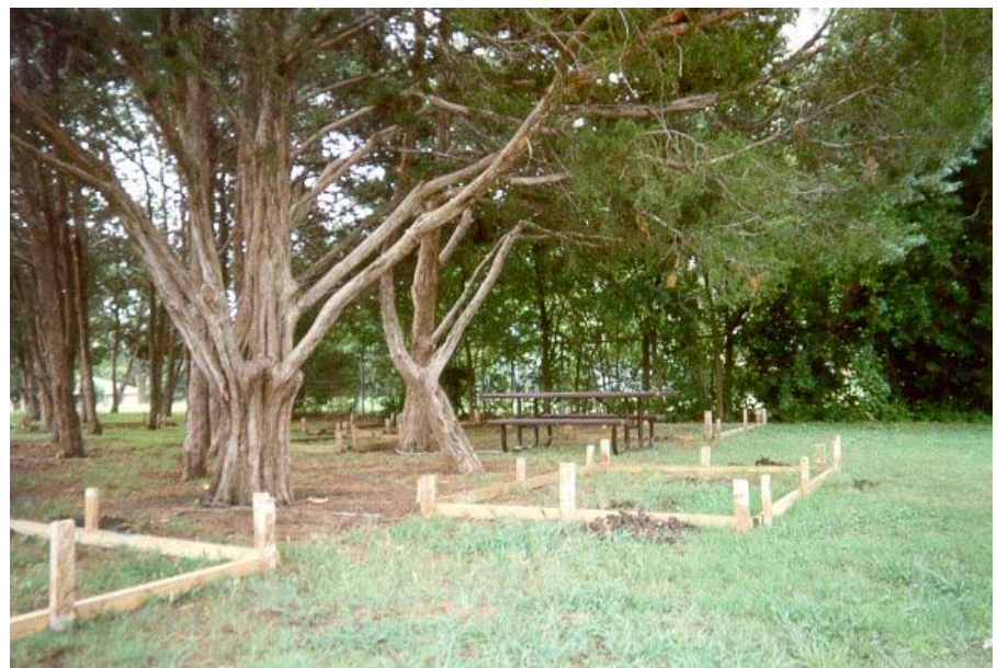
Installation of new benches, picnic tables and trash receptacles continues at Moss Park.
